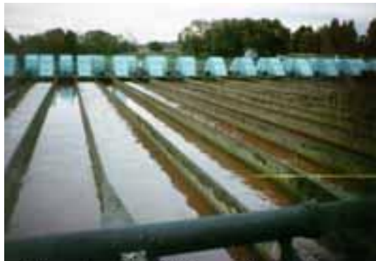
Figure 3 Sheffield aeration system at Stockport WWTP from 1924-1927.
